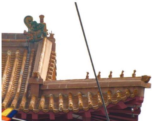
Figure 18: Application of imperial Chinese features in a recent Chinese structure in Melaka
